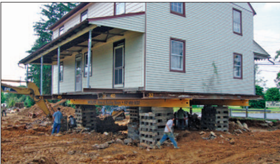
Figure 5R-8. Structure is separated from its foundation (photo courtesy of Wolfe House Movers)
