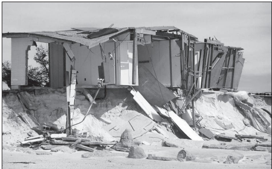
Figure 3-8. Large, fast-moving waves combined with erosion and scour to destroy this Gulf of Mexico home during Hurricane Opal
