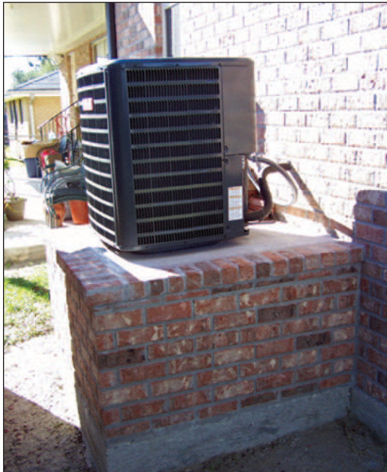
Figure 5W-1. Elevated air conditioning compressor
