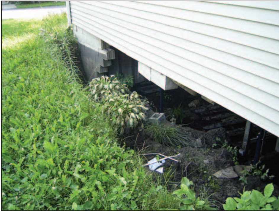
Figure 5D-29. Foundation wall failure due to pumping out basement while ground was still saturated with water
