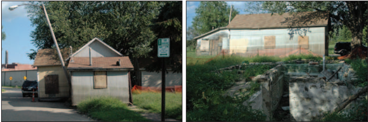
Figures 5D-11 and 5D-12. This house located in the SFHA was displaced from its foundation into the roadway adjacent to it. The photo on the right shows the house's original location.
