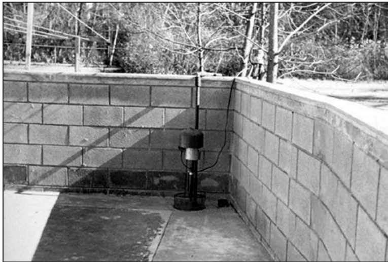
Figure 6-54. Interior sump pump for a residential floodwall
