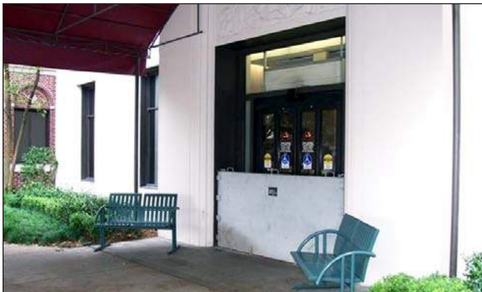
Figure 6-41. Example of a flood shield over a door
