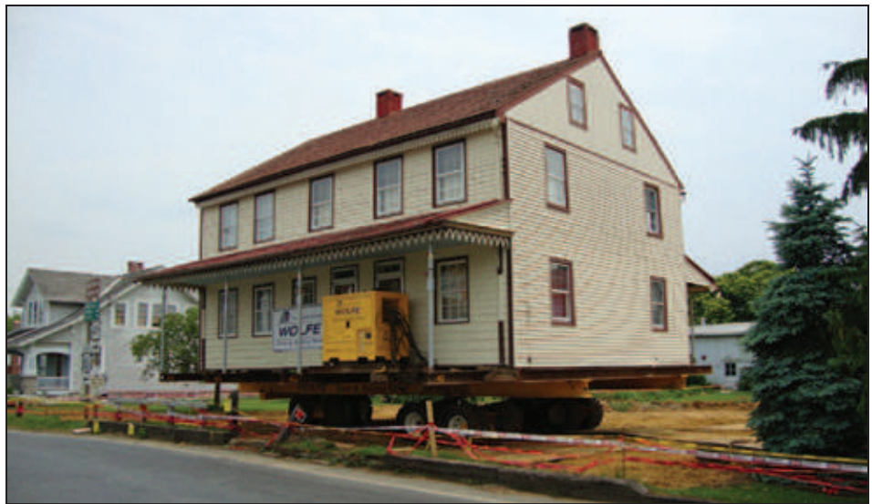
Figure 5R-12. Trailer is used to pull the house to the street (photo courtesy of Wolfe House Movers)
