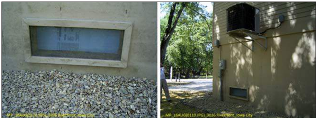
Figure 5E-14. A house where flood openings have been covered by insulation and drywall
