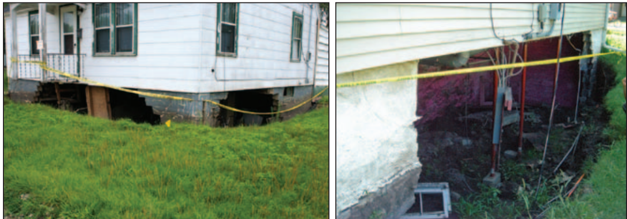
Figure 5D-14. This house’s foundation walls were not able to withstand the forces applied during or after the flood. Rebar would need to be added to help with reinforcement of the CMU foundation.
