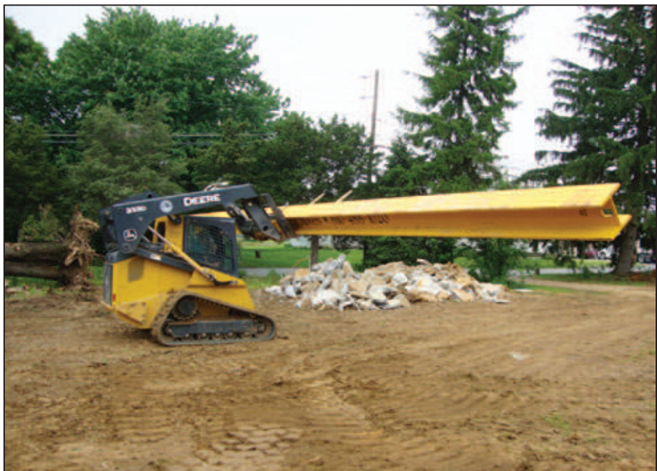
Figure 5R-9. Foundation preparation at new site (photo courtesy of Wolfe House Movers)
